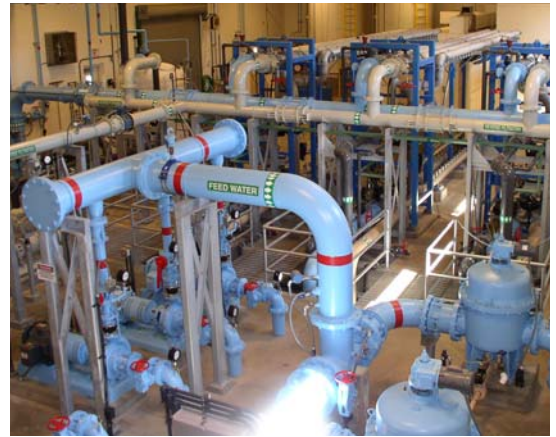
Inside the new Buckhorn Water Treatment Plant that serves approximately 3,500 customers.
