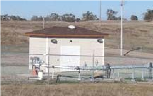
An new well and intertie system provides strong producing wells, reliability and flexibility for the customers of Camanche.
