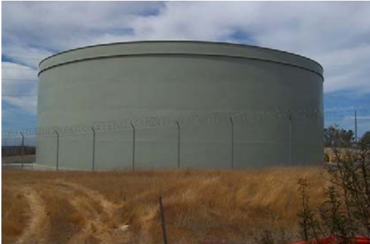
The two-million gallon Wildflower Water Storage Tank comes at no cost to existing customers.
