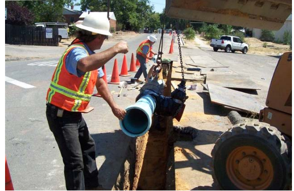
The Agency was able to upgrade an existing water main to increase fire flows and water source for Lone.
